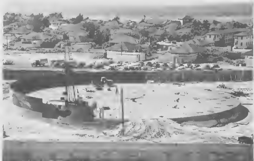
4 STEEL FLOORING is laid on the sand, and welded to the first row of plates in the wall—the first "shell course." VLOER DI Staal ta worde poni ariba e santo, y geweldo na e promer fila di plachi den e muraya — e promer "shell course."
